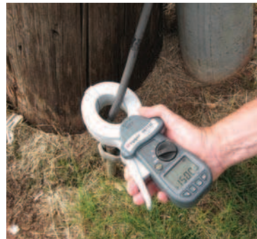
The DET14C is being used to test a pole ground.
